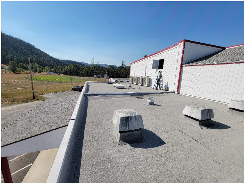
Figure 2: Roof Above Entrance Showing Roof Steps
